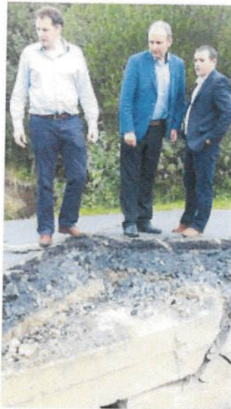
FF leader Michael Martin, TD, Charlie McConarogue and Cllr Martin McDermott survey the road damage yesterday. (North West Newsport)
